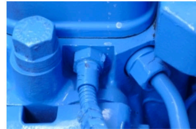
boudin emergency generator
